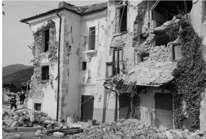
Figure 3.3: Damage found in a building aggregate in Castelnuovo village, belonging to San Pio delle Camere municipality.
