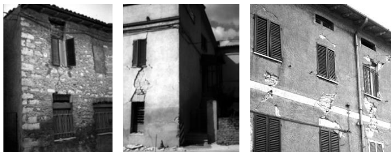
Figure 3.12. Some examples of earthquake damage in existing unreinforced masonry buildings (Cattari and Lagomarsino, 2008).
