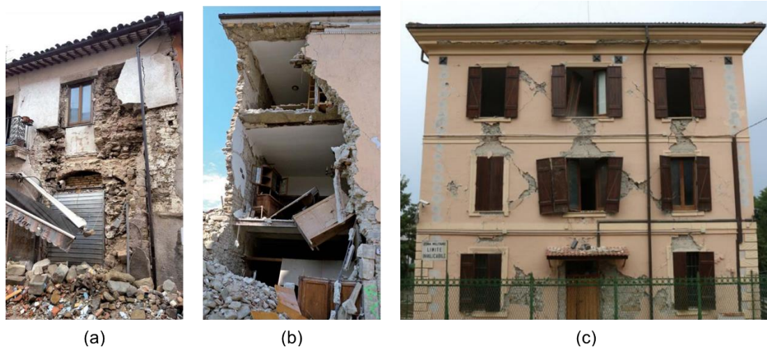
Figure 1.3. Damages from past Italian earthquakes to URM structures: (a) crumbling of the masonry, (b) Out-Of-Plane modes and (c) In-Plane modes (adapted from Fragomeli et al., 2018; Santarsiero et al., 2016).
