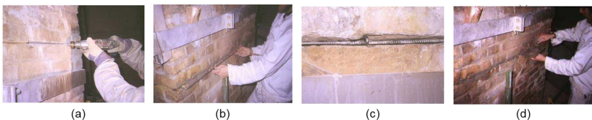
Figure 4.19. Reinforced repointing: (a) make holes drilling, (b) positioning of the transversal steel tie, (c) detail of the transversal steel tie (d) finishing of the intervention (adapted from Valluzzi et al., 2004).
