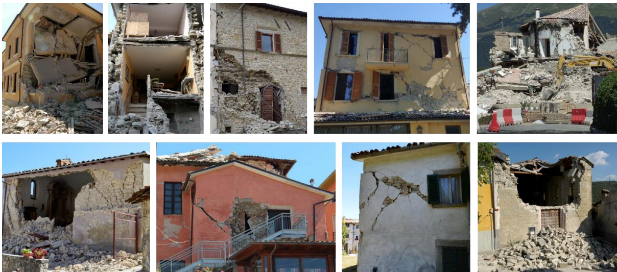
Figure 1.2. Several and different types of damages observed in URM structures after Central Italy earthquake of 2016 (adapted from Menna et al., 2016).
